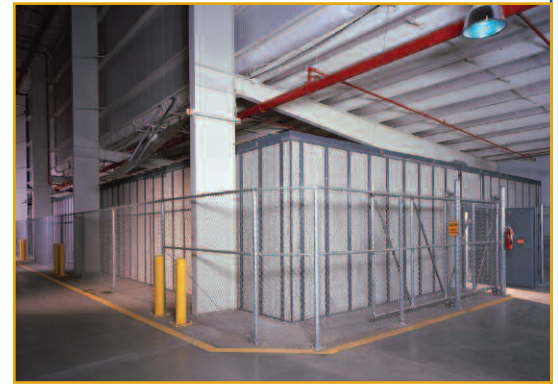
Exterior view of a newly-installed Firelock media storage vault.
